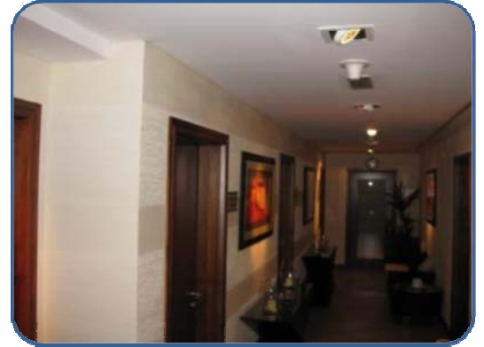
Hallway with ceiling mounted CellMax-0-25 Antenna
